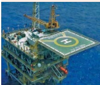
Rashpetco's P1 unmanned platform, Rosetta.
