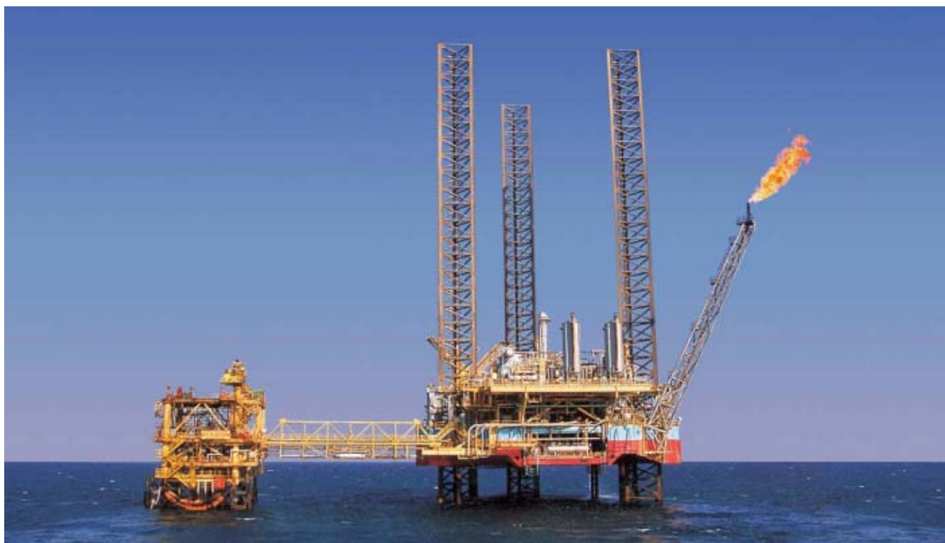
View of Geisum offshore platform, Gulf of Suez. Most of Egypt's natural gas reserves lie in the deep and ultra-deep water.
