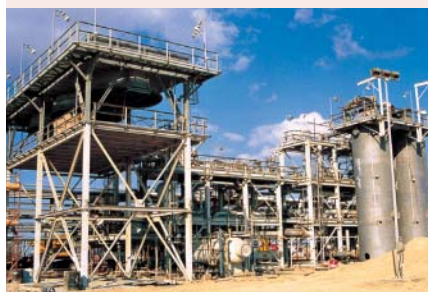
Gas treatment station at Rashid Area.
