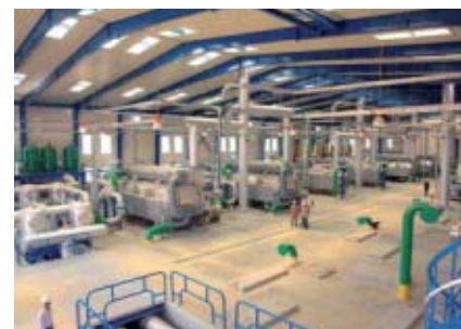
Cooling and heating station, Gas Cool Co.
