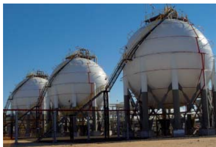
UGDC gas storage tanks.
