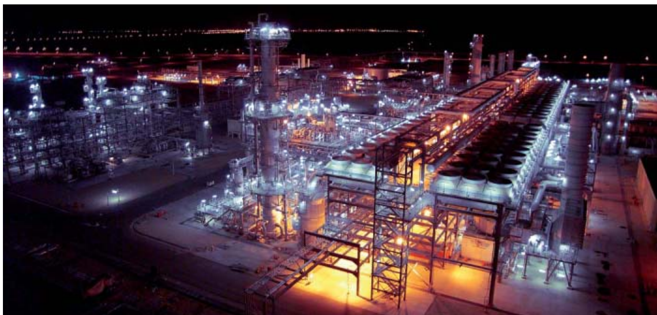
A big part of world's energy future belongs to natural gas. View of LNG plant in Mubarak Complex for Natural Gas and Petrochemicals, Damietta .
