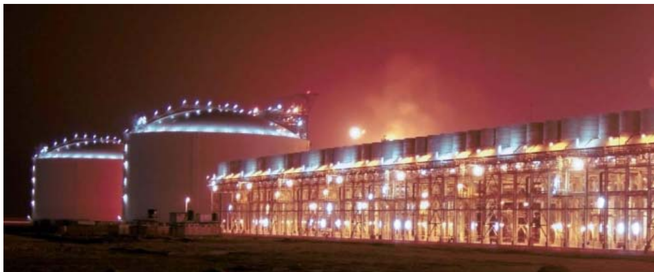
Enhancing the capacity of Egypt's gas grid will accommodate growing demand for natural gas. View of storage tanks in LNG plant.
